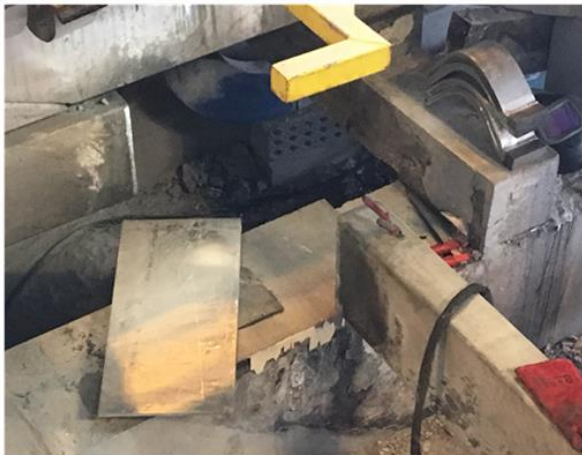
Figure 7. Bus bar prepared before welding (damaged part has been cut off).
