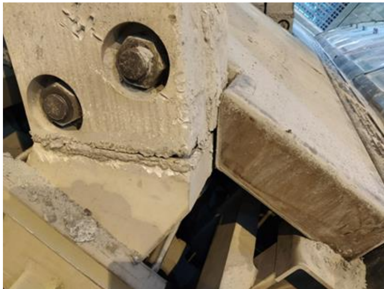
Figure 2. Example of broken weld on the middle riser.
